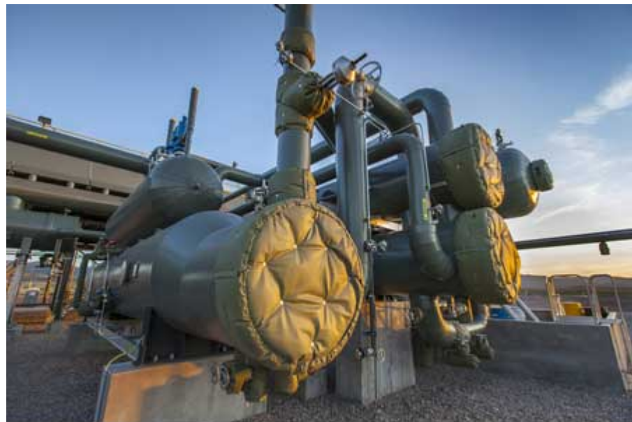
Veyo Heat Recover Plant
